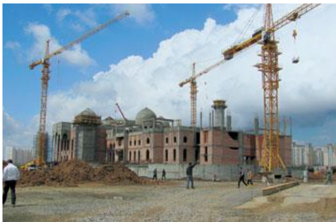
The largest mosque in Kazakhstan to accommodate more than 5,000 worshipers is being erected at an accelerated pace.
